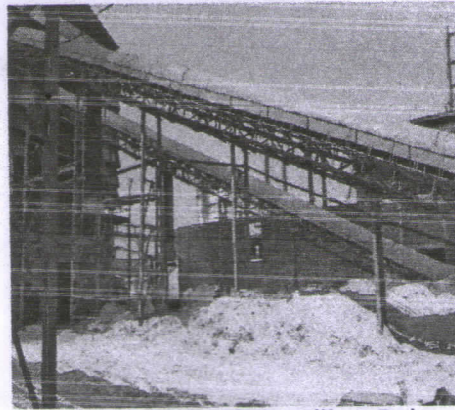
Fig-4 Boiler Fuel Handling Belt
